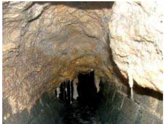
Fat beginning to block a sewer
