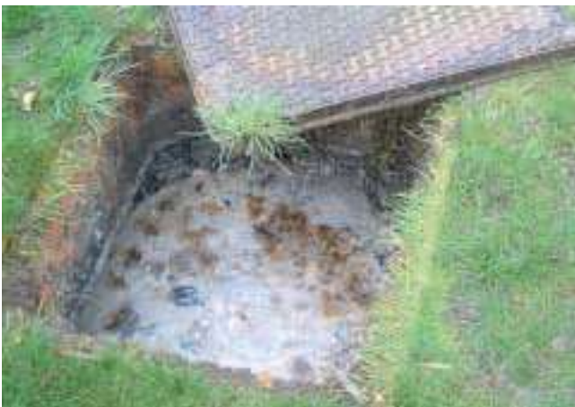
Fat building up in a manhole
